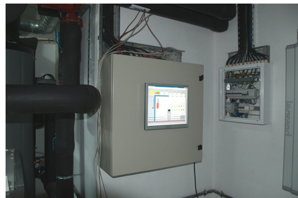
Fig. 8. GSHP Measurement and Control System of the GroundMed Coimbra demo site.
