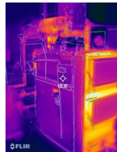
Fig. 3 – The entire boiler
