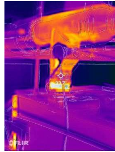
Fig. 8 – The flue gases duct
