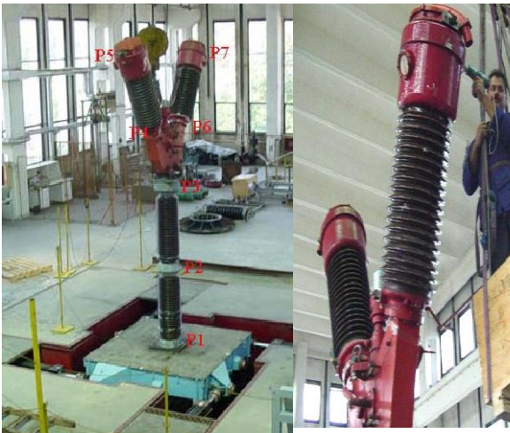
Fig. 1. Position of measurement and excitation points for IO 220 kV/2500A circuit breaker.
