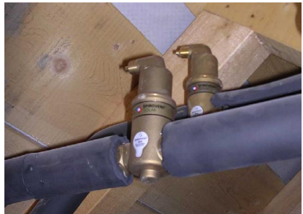
Fig. 10. Inappropriate components (automatic air vent) for venting the primary collector loop
