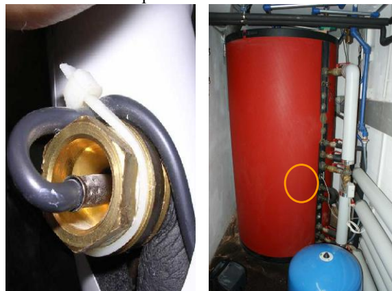
Fig. 19. Deficient sensor mounting (left) position of 'storage-bottom' sensor too high (right)
