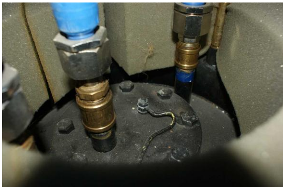
Fig. 13. Very poor heat storage insulation at the top of the tank, which is the hottest place.
