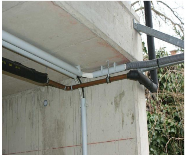
Fig.5. Partially missing pipe insulation, no protection against animal bites and UV radiation
