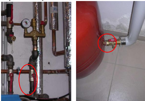
Fig. 8. Pressure control valve (left) and membrane expansion vessel (right): may both be blocked
