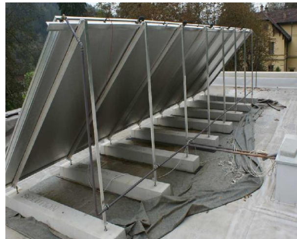
Fig. 6. Pipe insulation missing from solar circuit external pipes
