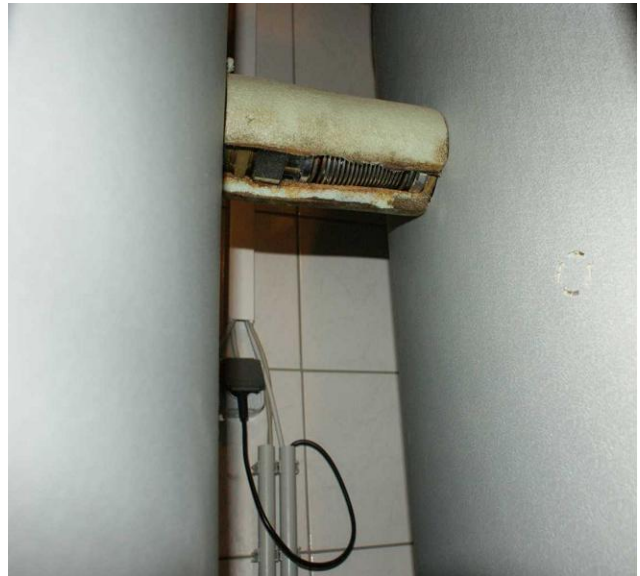
Fig. 15. Inappropriate insulation material which did not survive the high temperatures which were reached in the heat storage.
