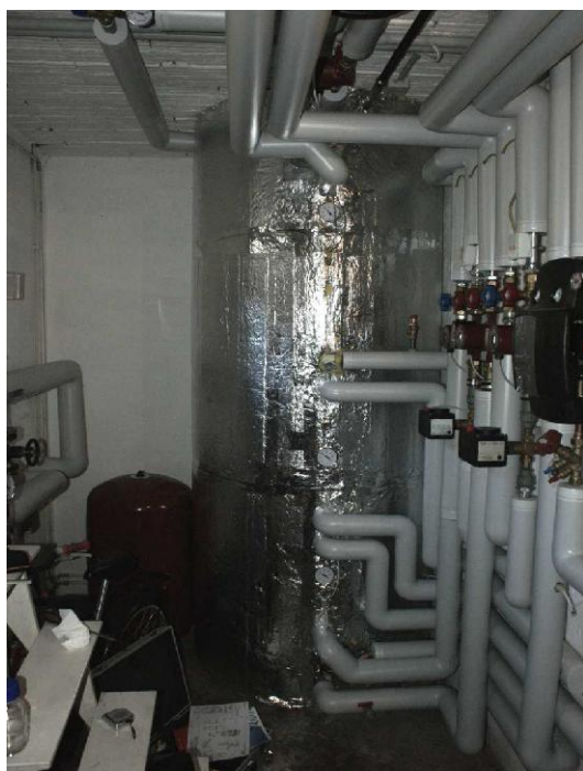
Fig. 17. Additional insulation on top of the standard insulation, connections insulated up to storage tank insulation
