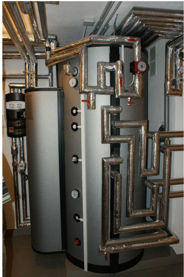
Fig. 16. Storage tank with exemplary good thermosiphon heat trap installation of the pipe connections.
