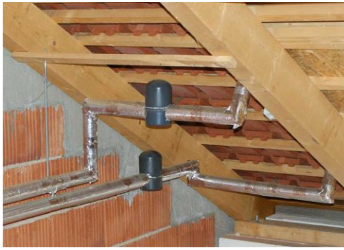
Fig. 12. Example of correct chosen manual maintained air vents which are insulated and withstand also high temperatures; perfect rock wool insulation of the pipes.
