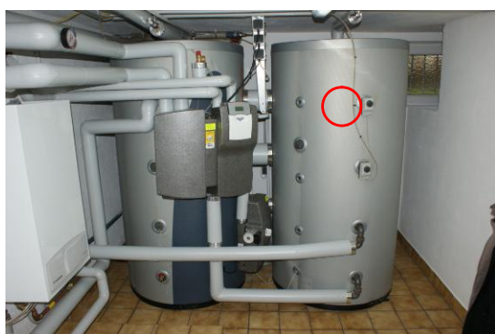
Fig. 18. Flow pipe connection for DHW preparation from the tank on the left side, but sensor for auxiliary heating of the tanks on the tank on the right side leads to long delay in reaction of auxiliary heating.
