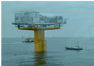
Figure 4.2 Offshore transformer station
