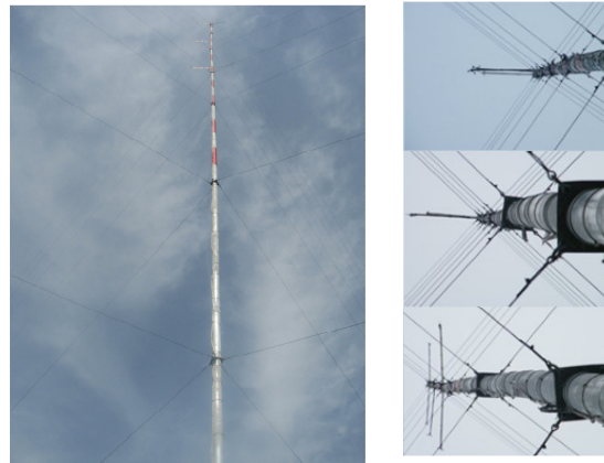
Fig. 3. Wind tower fully equipped
