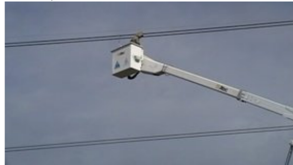
Fig. 9. Live working method – bare-hand method use insulating arm elevating platform truck with insulating arm, presented by SC SMART SA [7].
