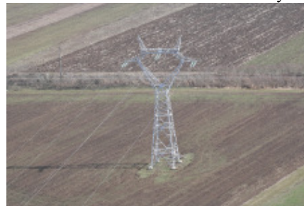
Fig. 1. An overview from the multispectral inspection of tower of OHTL is shown in the visible spectrum [1].
