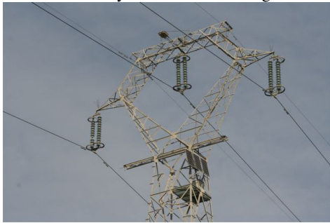
Fig. 7. Monitoring system on OHTL is shown [3].
