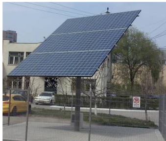
Fig. 1. View of LACARP PV system
