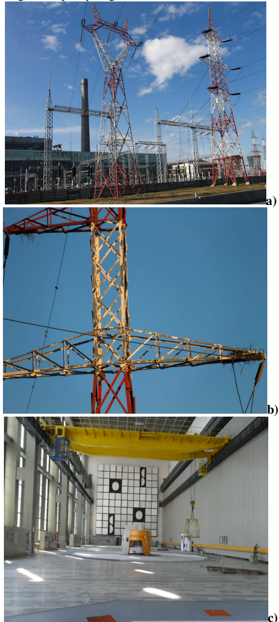
Fig. 1. (a) Electro-energetic installations exposed to corrosion in complex polluted environment (b) Installation exposed to atmospheric corrosion in open spaces (c) Electro-energetic installations exposed to atmospheric corrosion in indoor spaces.
