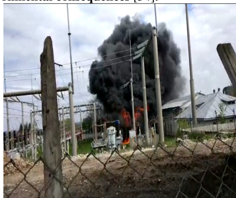
Fig. 1. Explosion and simultaneous incineration of several transformers in Botosani (RO) [31]
